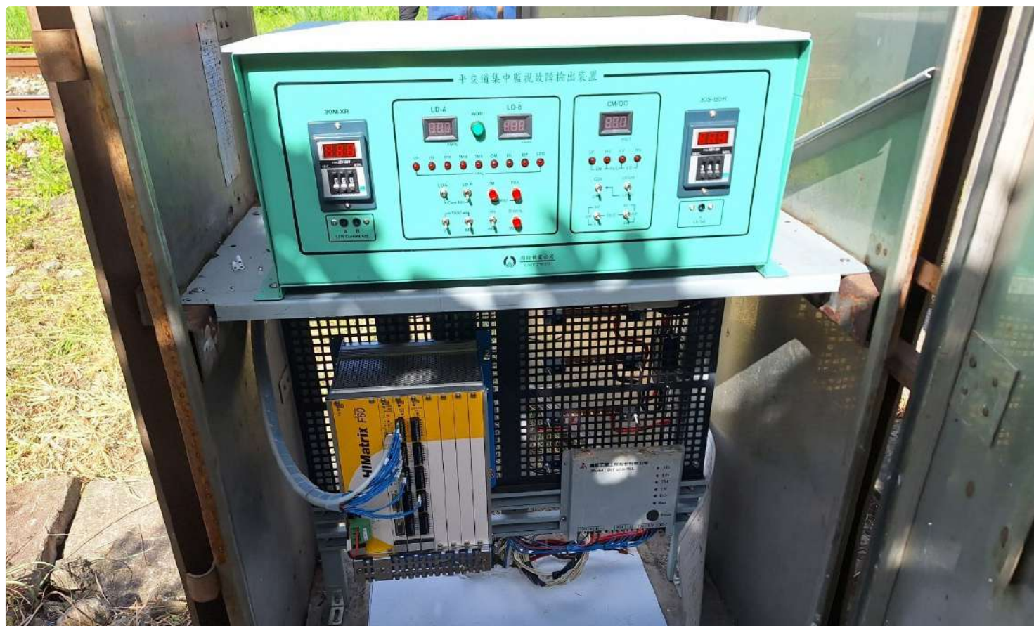
Centralized Monitoring Terminal (CMT) for Level Crossing Fault Detection
