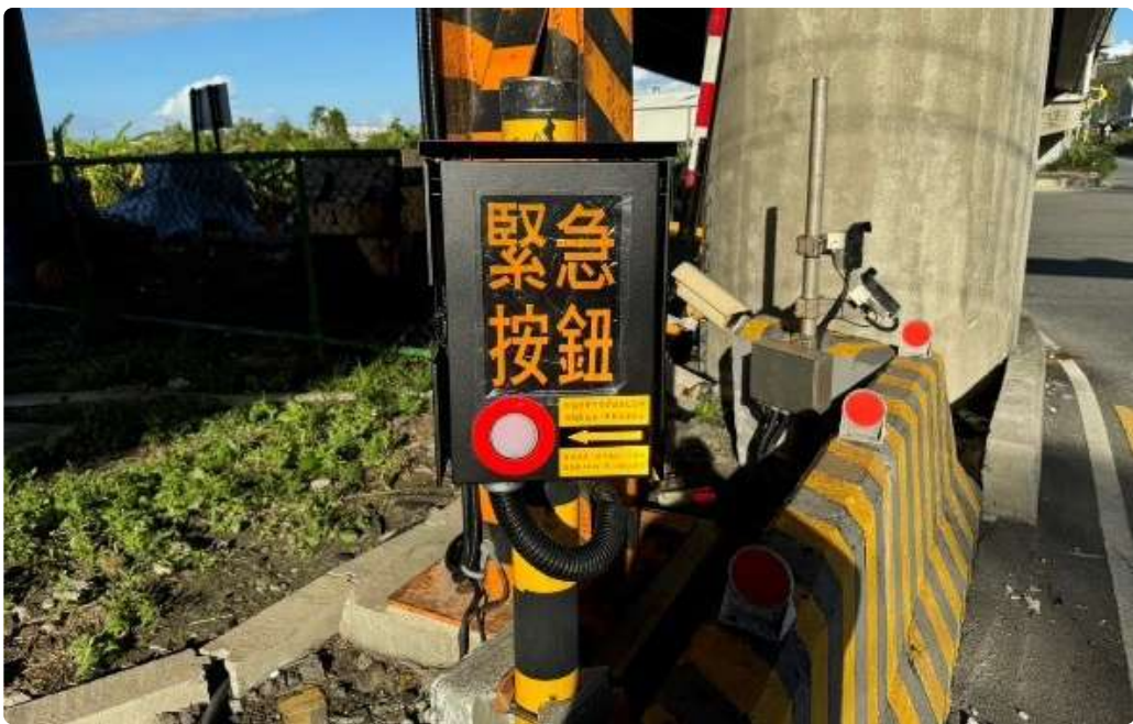
Updated Manual Emergency Button at Level Crossing Entrance
