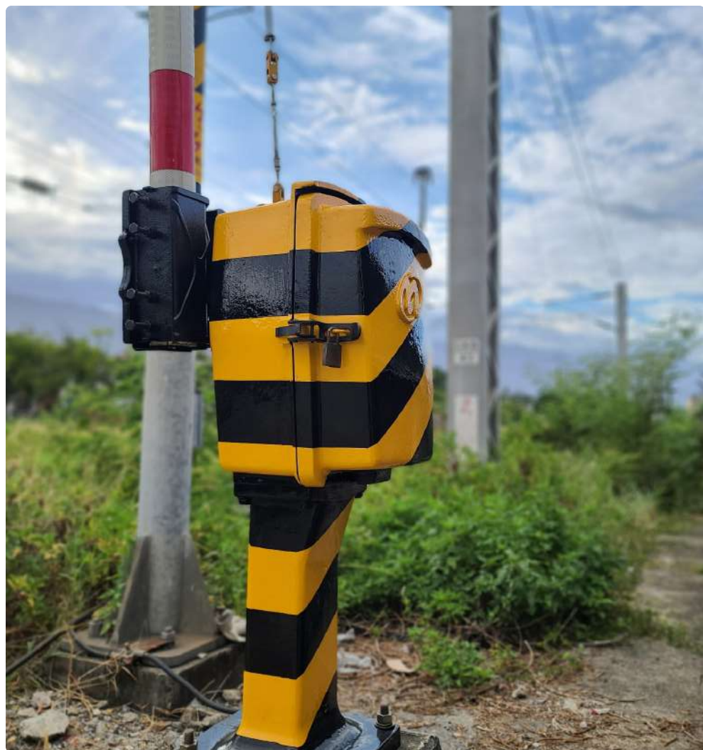
Overall Exterior View of the Barrier Unit
