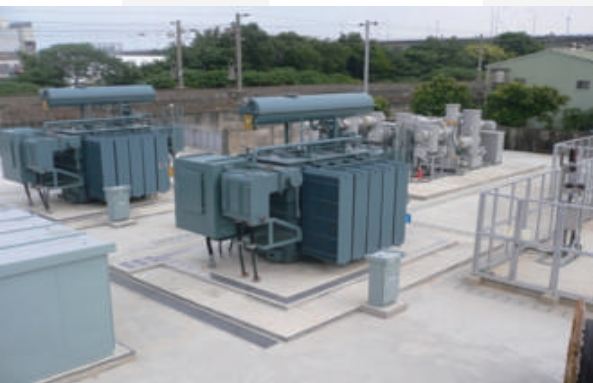
上圖為容量擴增為50MVA變電站 The picture above shows the substation with power capacity increased to 50MVA.
