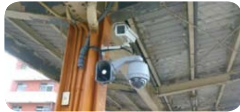
車站錄影監控設備 Video surveillance system equipment at a TRA station
