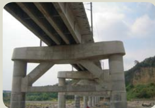
完成臺中線大甲溪橋橋基換底工程 Completed foundation replacement for Dajia River Bridge in Taichung Line
