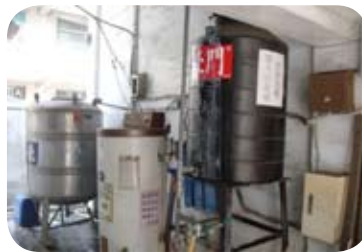
逆滲透及回收處設施 Reverse osmosis fountain and recycling station
