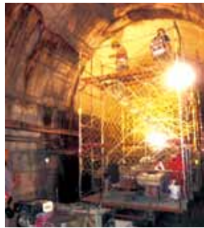
▲ 南迴線枋野三號隧道辦理裂縫止水補強灌漿 Fangye Tunnel No. 3 in South-link Line Water retaining reinforcing grouting
