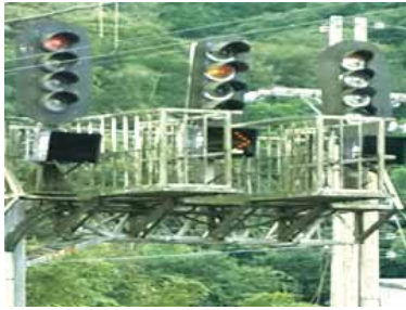
▲ 軌旁號誌機設備 Signal equipment
