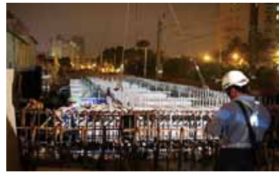
▲ 鐵路臨時鋼橋工程 + 600 in South-link Line Construction of a temporary steel bridge for the railway
