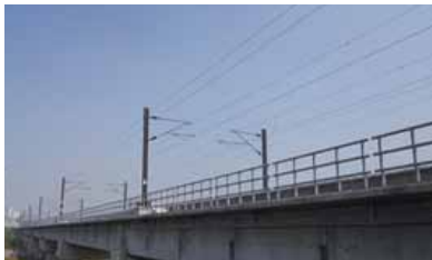
◀ 二層行溪橋改建工程完工 River Bridge Completion of Ercengxing River Bridge
