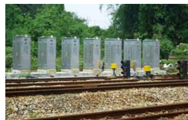
▲ 軌旁號誌繼電器箱設備 Signal relay equipment
