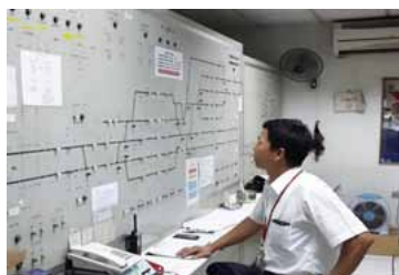
▲ 號誌聯鎖就地控制設備 Signal interlocking control equipment
