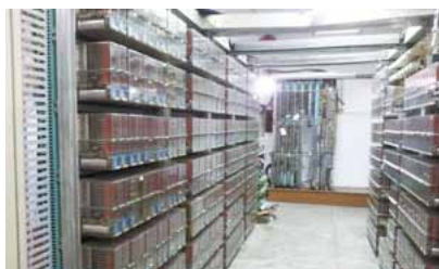
▲ 號誌聯鎖系統設備 Equipment of signal interlocking system
