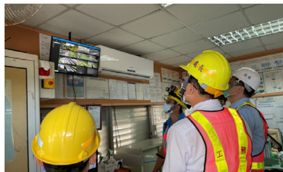
Equipment in the front and rear station operation rooms
