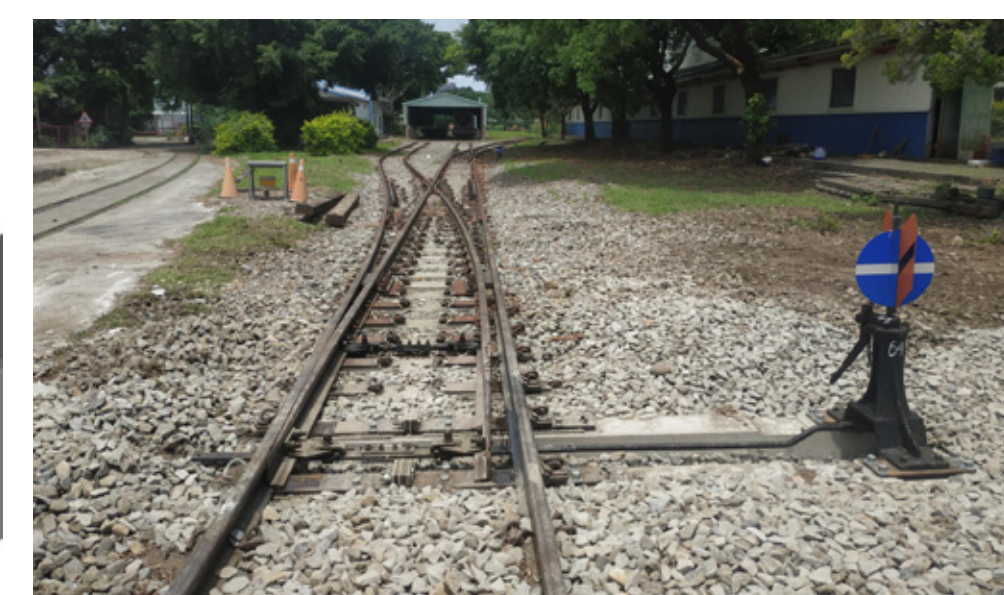
Image ⑧ Actual laying This case, from problem discovery, investigation and analysis, discussion and improvement to design drawings, was completed by colleagues from Taiwan Railway Administration. Related parts were produced with the cooperation of domestic manufacturers. They were laid on the track of the maintenance team in May 2023.
