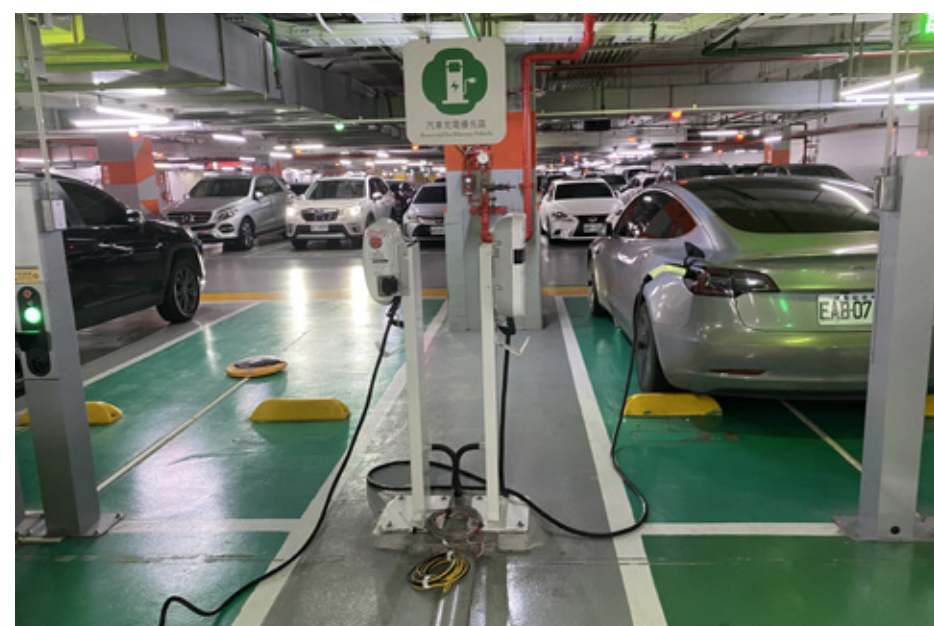
Taipei Station underground parking lot charging station
