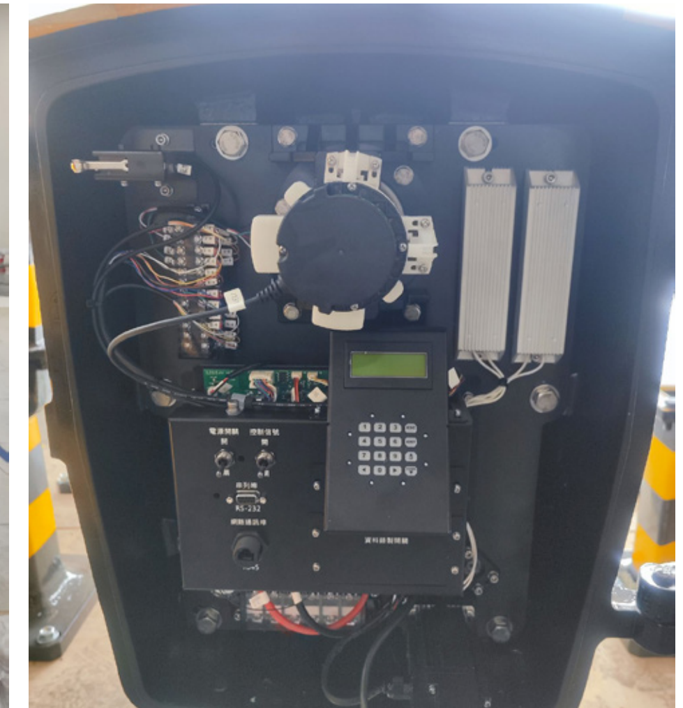
Internal view of the controller of crossing barrier
