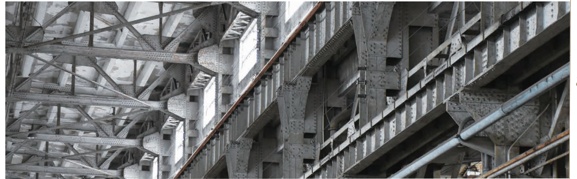
組立工場鋼架上密密麻麻的鉚釘，都是以嵌入熱擊法鉚接，因此十分堅固 Steel frames at the Erecting Shop are studded with rivets, which are tempered for strength.
