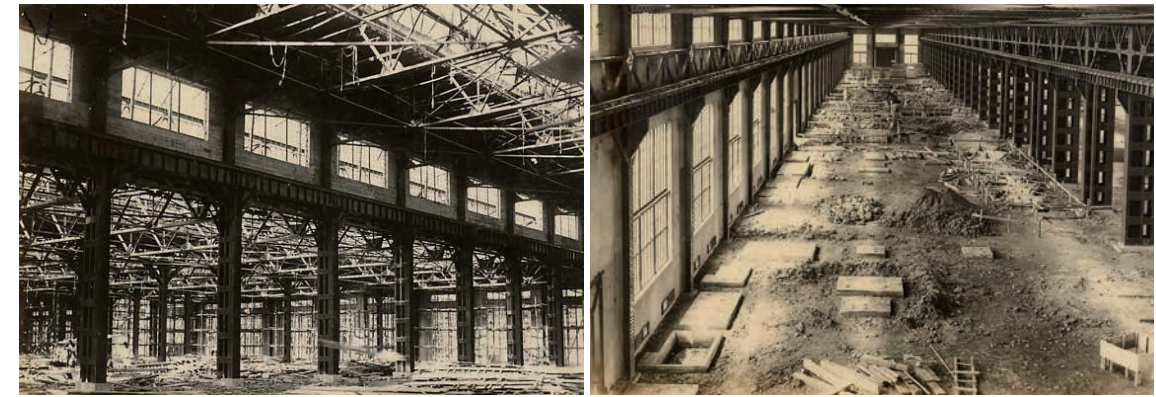
車輛場區（左圖）及機器工場內部的鋼架結構，氣勢驚人，是當代工業建築的典範 The rolling stock area (left) and machine shop are both breathtaking in size, and were archetypes for their time.
