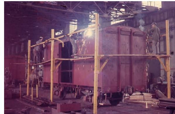
泰國守車車架電焊作業 Electric welding on caboose frames destined for Thailand.
