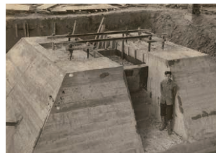
完成混凝土作業的廠房基座 The reinforced concrete base is completed.
