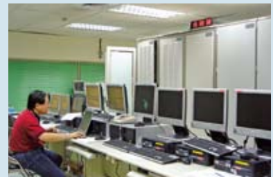
行車調度無線電話系統中央調度設備 Central dispatch equipment of the train dispatch wireless phone system
