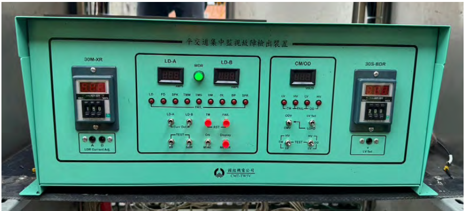
Centralized Level Crossing Monitoring Equipment and Transmission/Receiver System (CMT) Fault Detection Unit
