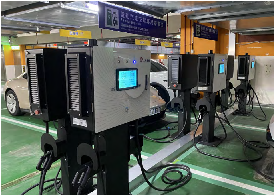
Nangang Parking Lot 1-Fast charging ports
