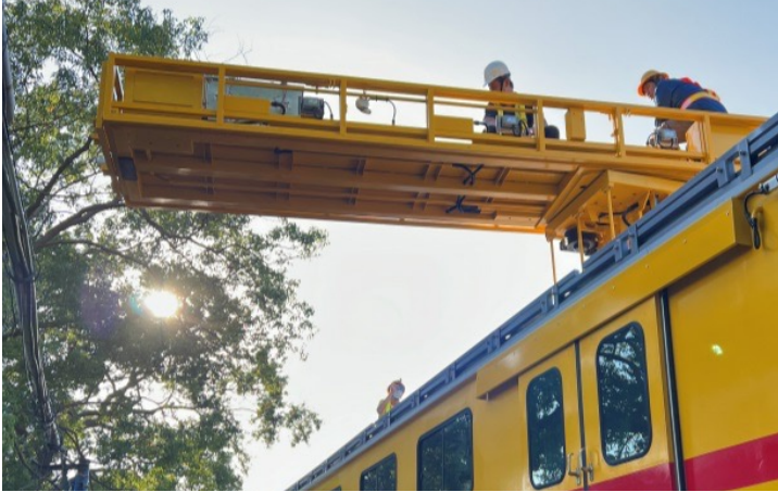
The platform of the Overhead Catenary System (OCS) motor car is being tested using weights to assess its load-bearing capacity
