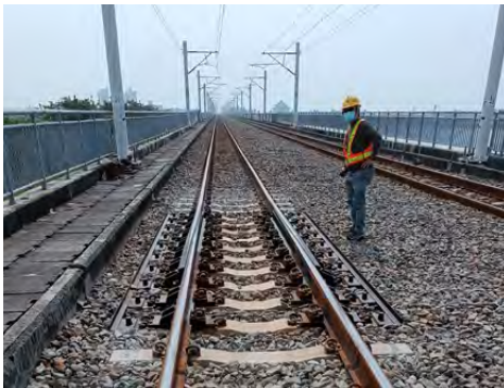
Continuous welded rail (CWR) with expansion joints installed at both ends to accommodate rail movement.
