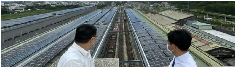
Chairman Tu Wei conducted an inspection of the solar photovoltaic equipment.
