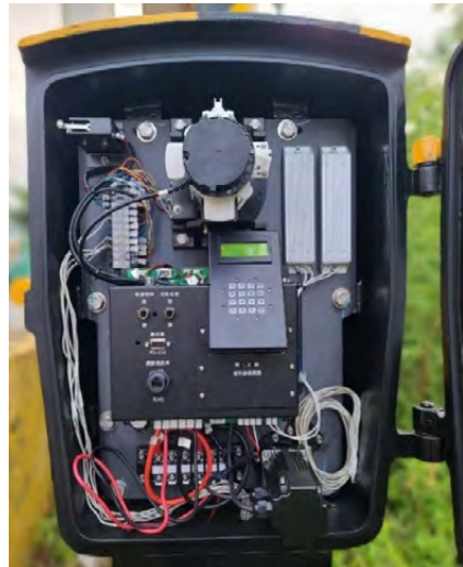
Full internal view of the barrier gate
