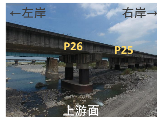
P26基礎裸露深度約1.15m
