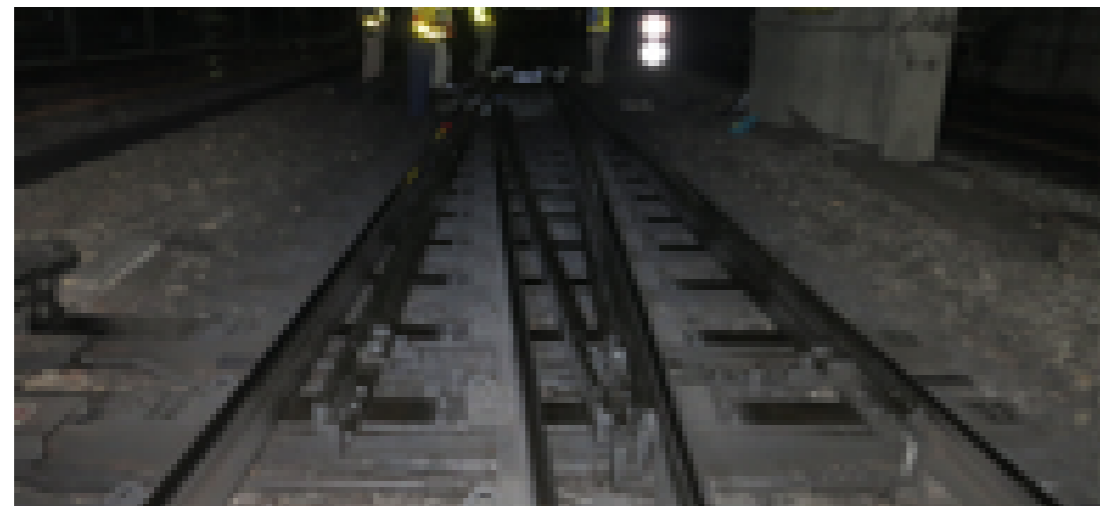
DSS of Taipei Station
