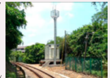
Radio base station of National Museum of Marine Science & Technology
