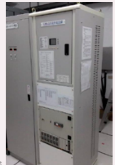
Switching the DC power supply system devices of Hualien electrical depot
