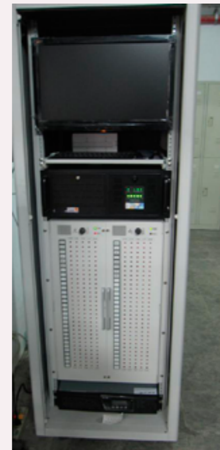
New level crossings monitoring system at the sub stations of Houlong
