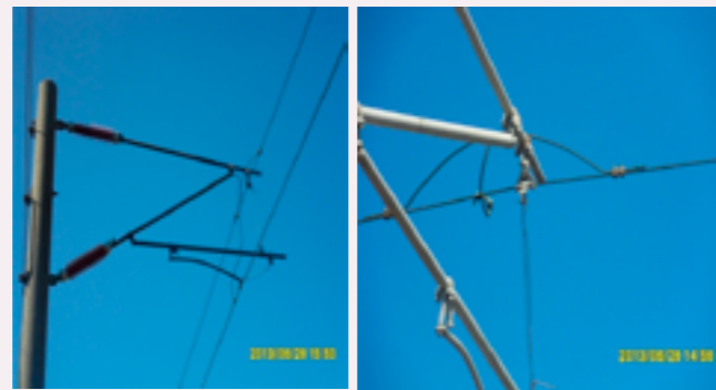
Messenger wire added with auxiliary line
