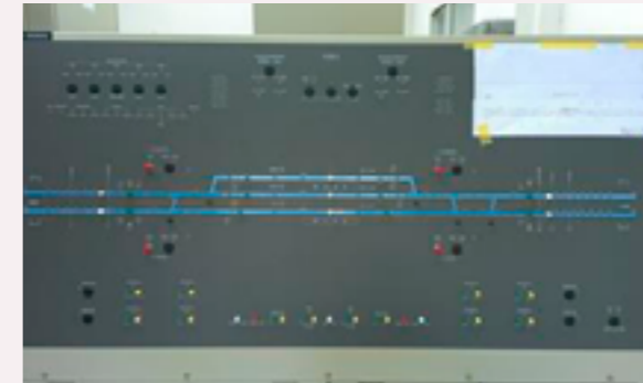
Upgraded signaling system to electronic interlocking in Taoyuan's temporary station
