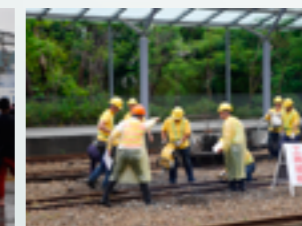
Line construction recovery drill as part of the railway safety drill in Alishan forest railway on May 26, 2015
