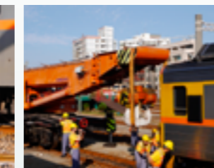
88-ton crane repair drill as part of the central region's railway safety drill on October 23, 2015
