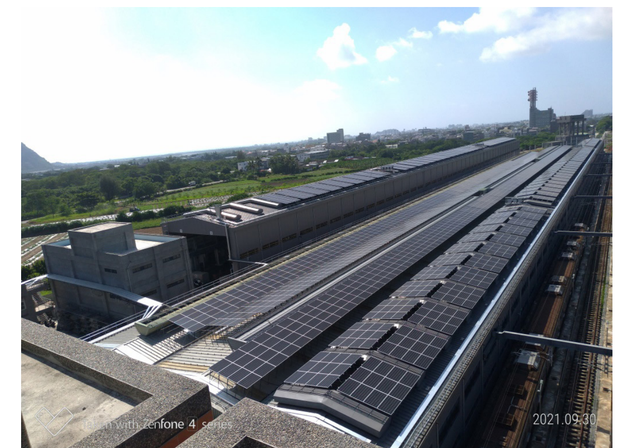
Solar photovoltaic equipment on roofs of maintenance garage of Taitung Rolling Stock sub-branch
