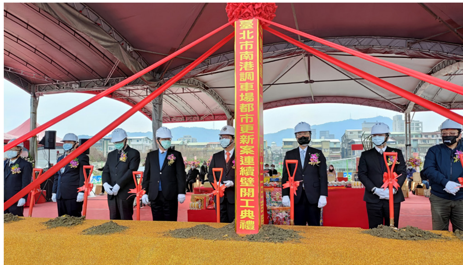
Commencement for construction of the diaphragm wall of Nangang Marshalling Yard Urban Renewal Project
